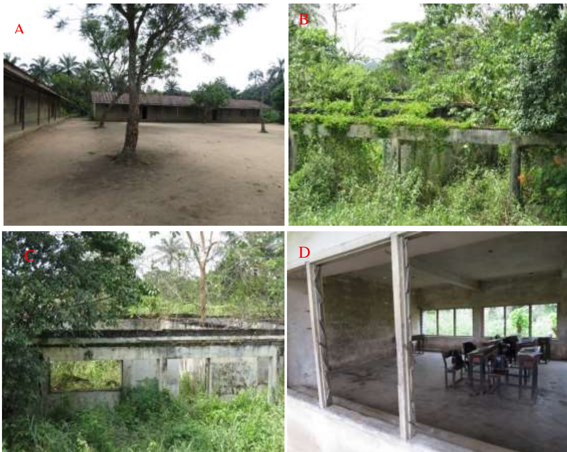
Figure 1. Infrastructural facilities: (A): Igbodo-Etche community primary school built by community effort. (B) Abandoned school building overtaken by grass and bushes. (c) Laboratories also overtaken by grass and bushes. (D) Dilapidated classroom in Ndashi Government Secondary School, Etche.
